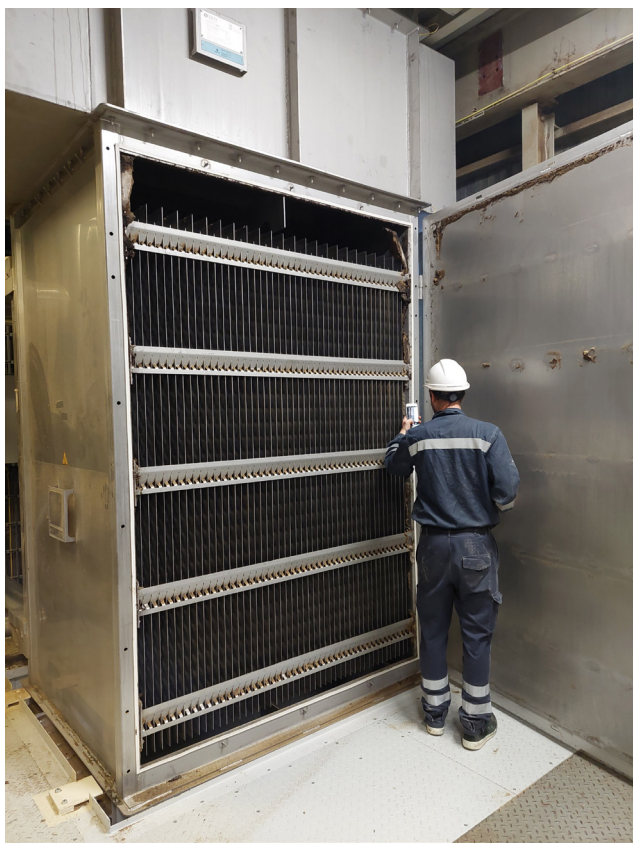
Figure 2. MBHEs and common trouble areas such as the heat exchange plates should be regularly cleaned and inspected.
