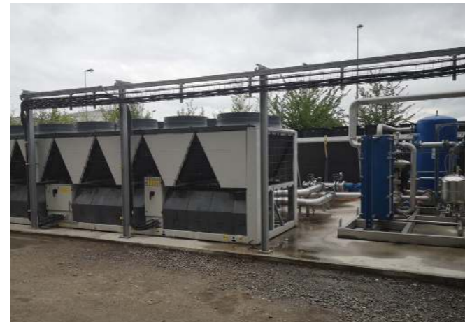
Figure 2: Chiller, Dry cooler and water module
