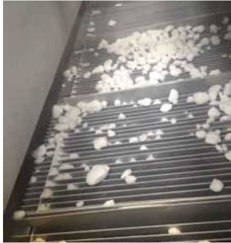
⚠ Agglomerated product that comes into the heat exchanger can lump on the tops of the plates and cause wear to the caps, as well as lead to blockages further down the unit.
